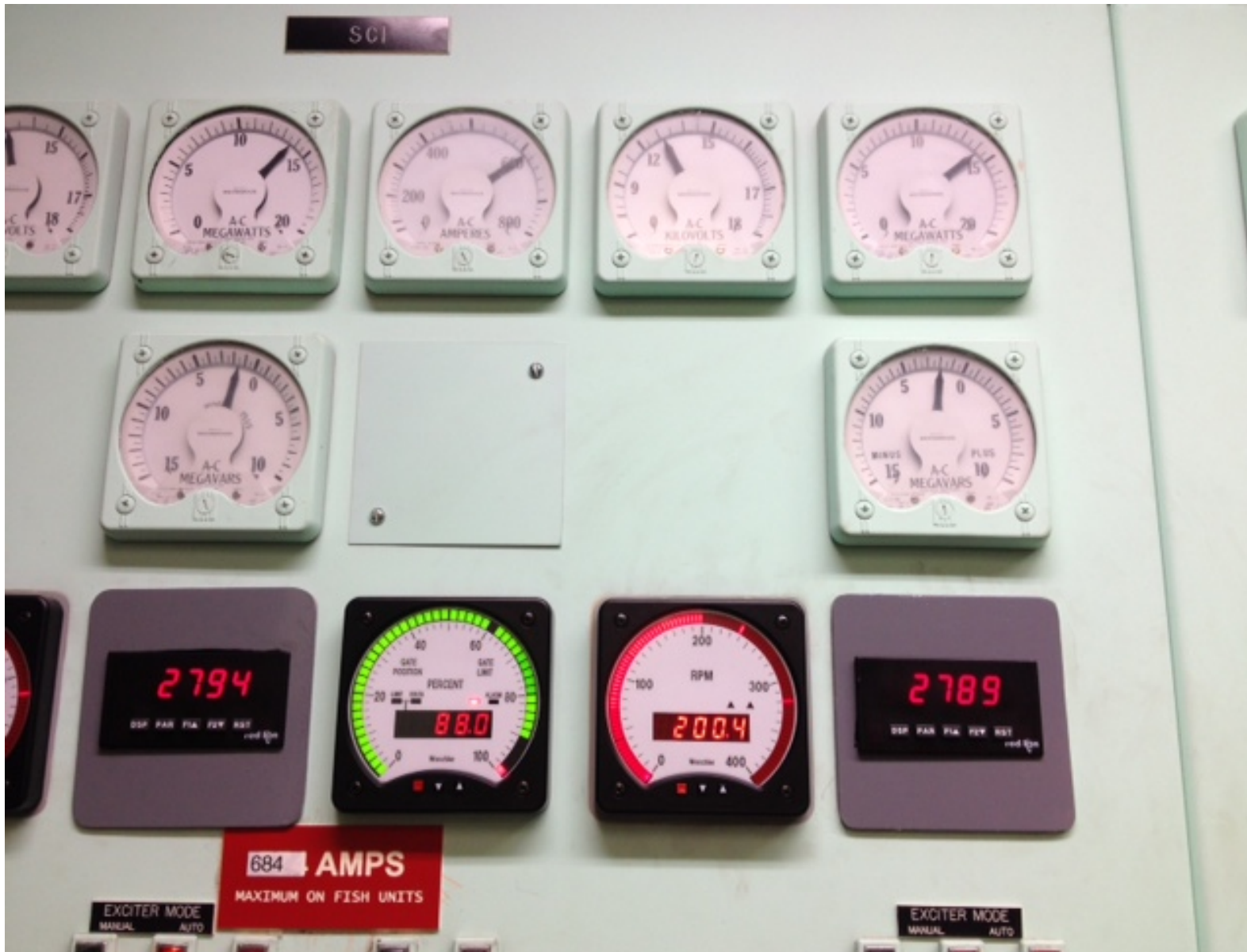
New fish unit governor upgrades provide automation by CFS rather than by prior Megawatt.
